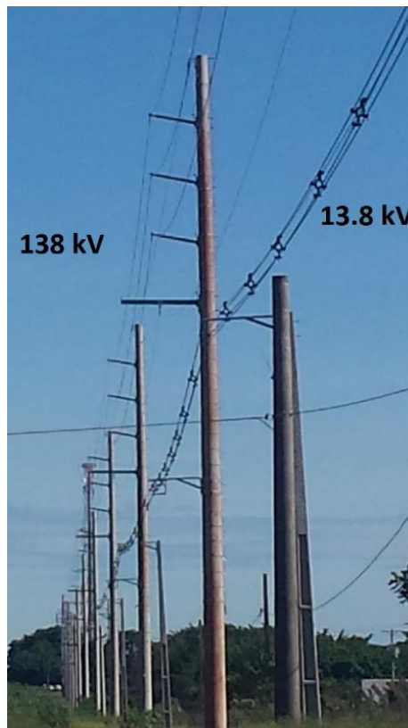
Fig. 1. Hybrid overhead line composed of 138 kV and 13.8 kV circuits (Campo Grande, Brazil), before the installation of the low-voltage circuit. (BATISTA MORAES et al., 2023)
