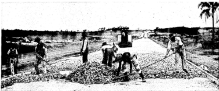
Workers laying crushed rock on a highway in the State of São Paulo, Brazil. Courtesy Office of Inter-American Affairs.
